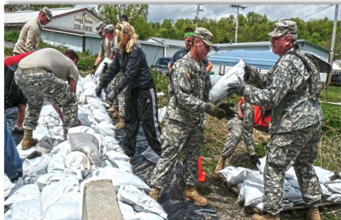
Soldiers of the 1140th Engineer Battalion, civilian first responders, and local residents work quickly to build a three-foot sandbag wall to prevent possible flood waters from closing a Missouri highway intersection. (Photo by Michelle Queiser/Missouri National Guard)
